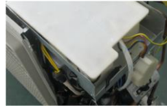
Sealed electric box
