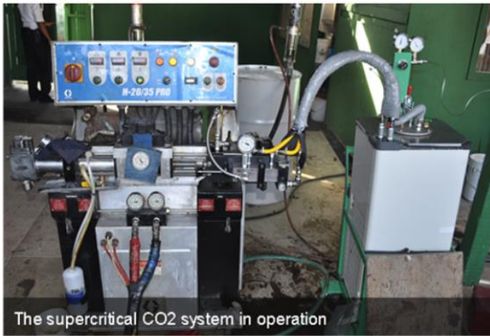
The supercritical CO 2 system in operation
