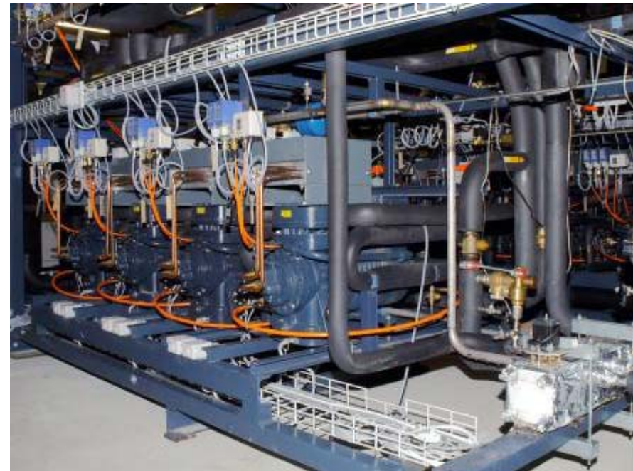
Prodega Basel, Switzerland medium temperature installation, Q'_0 = 80 \text{ kW}
