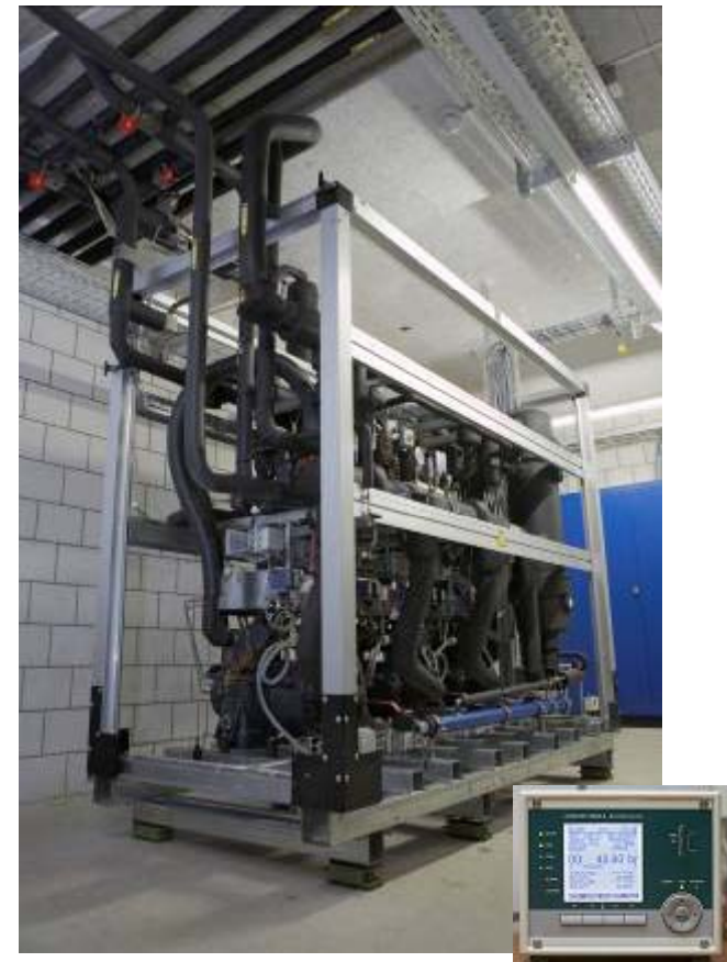
Growa Bern, Switzerland, low temperature installation, Q'_0 = 50 \text{ kW}
