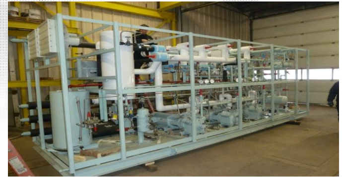
Energy Efficient Low Charge Ammonia CO2 Cascade System for Supermarkets
