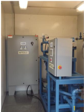
Controls and Access
