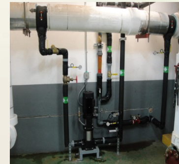
Heat Source Piping
