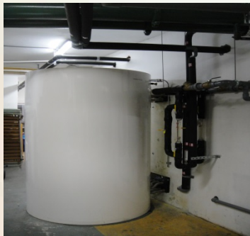
Hot Water Storage Tank
