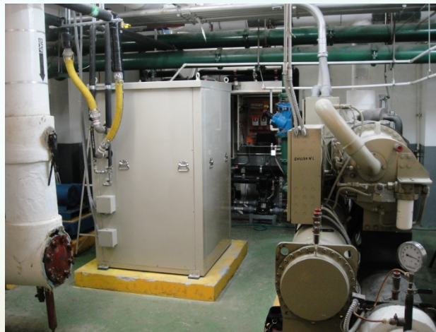
ECO Cute installed in chiller mechanical room
