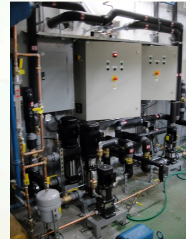
Hot Water Piping
