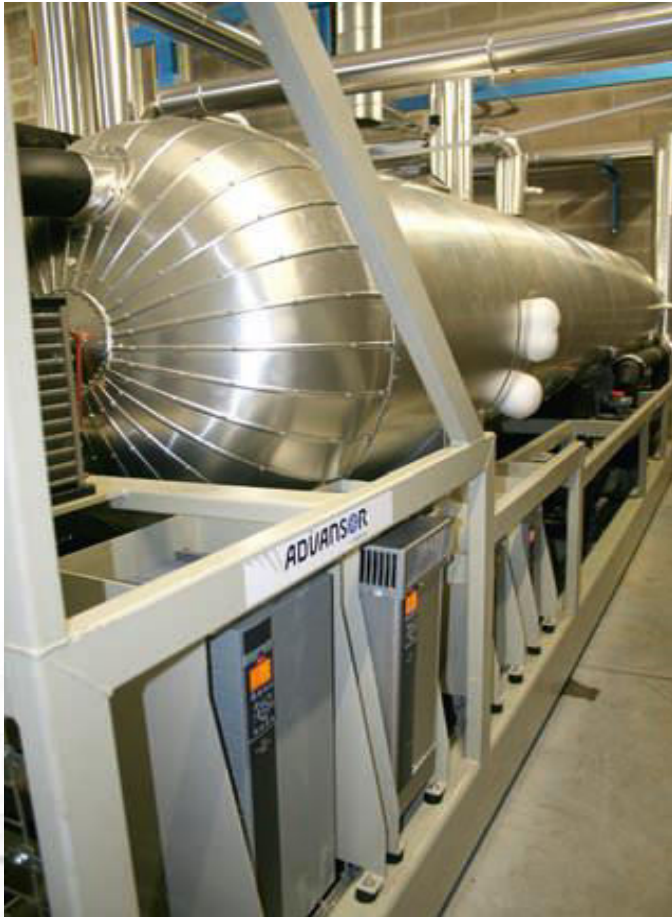
LT Vessel and inverter pumps side
