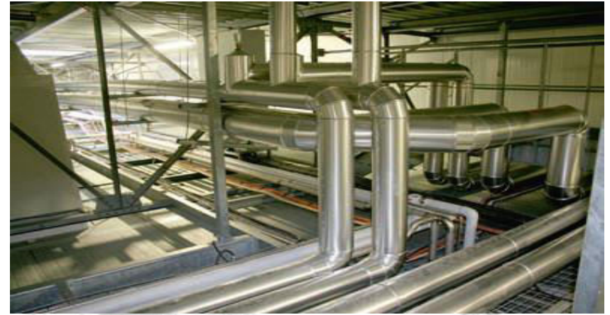
Loft piping CO2 & Chilled water
