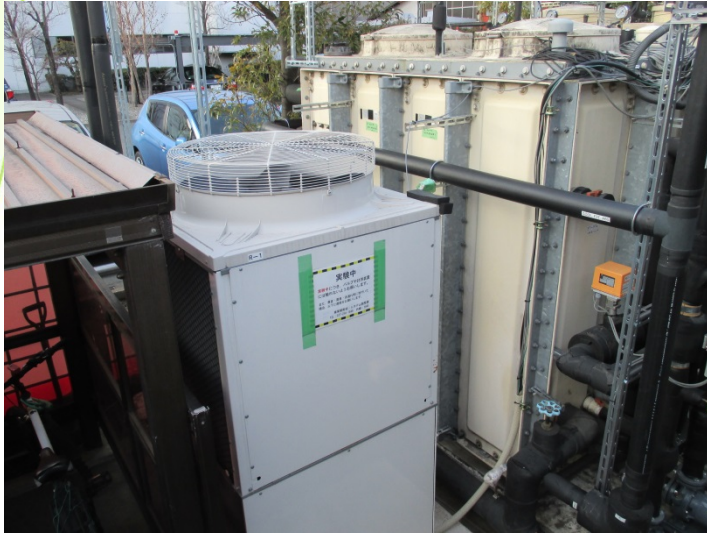
CO 2 refrigeration and storage tank
