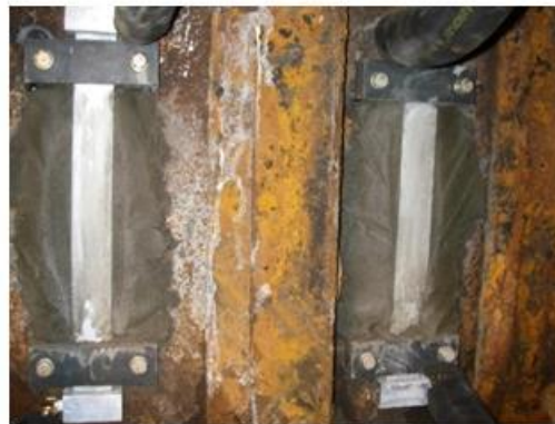
Freezing pipe attached at wall
