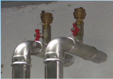
Additional safety installation
