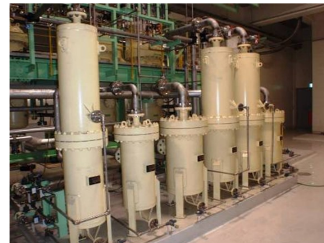
Filter Units for CO 2 Line
