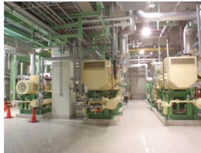
CO 2 /NH 3 Refrigeration Plant
