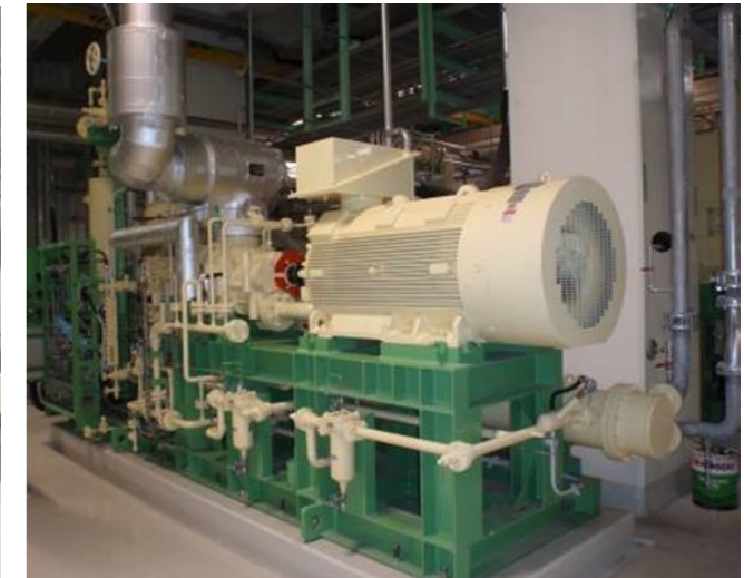
CO 2 Compressor Unit
