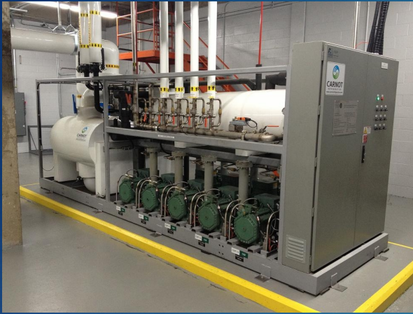
Large remote plant
