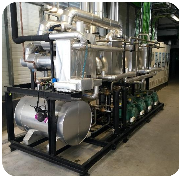
3 CO 2 Compressors rack
