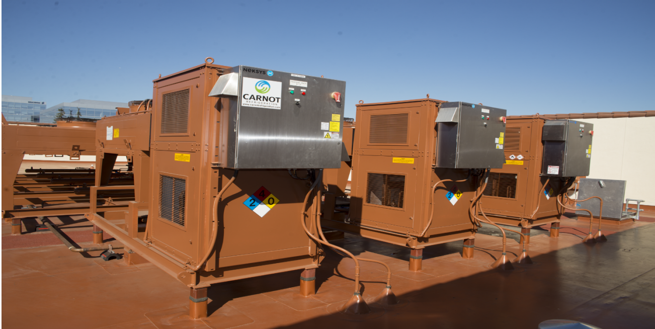
Three low-temperature propane chillers at Santa Clara store.
