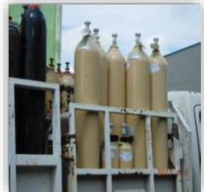
Storage at Coolcare's workshop (CO 2 gas)
