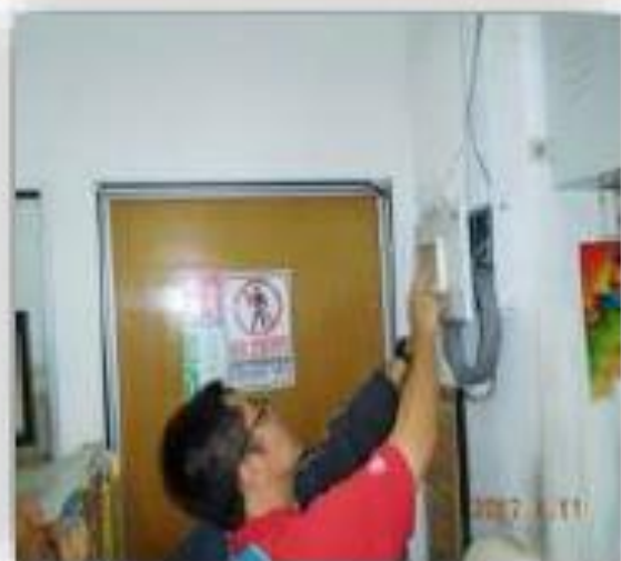
Setup controller system
