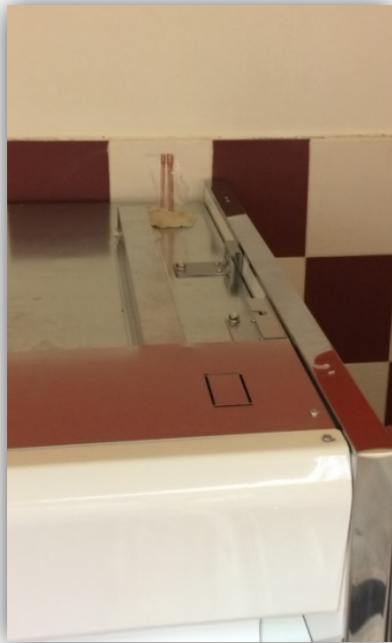
Piping outlet on top of showcase
