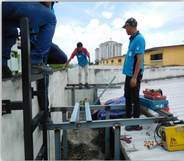
CO2 unit with platform
