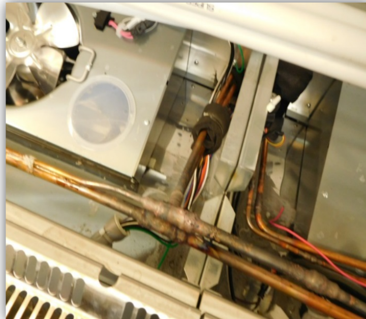
Piping connection inside showcase
