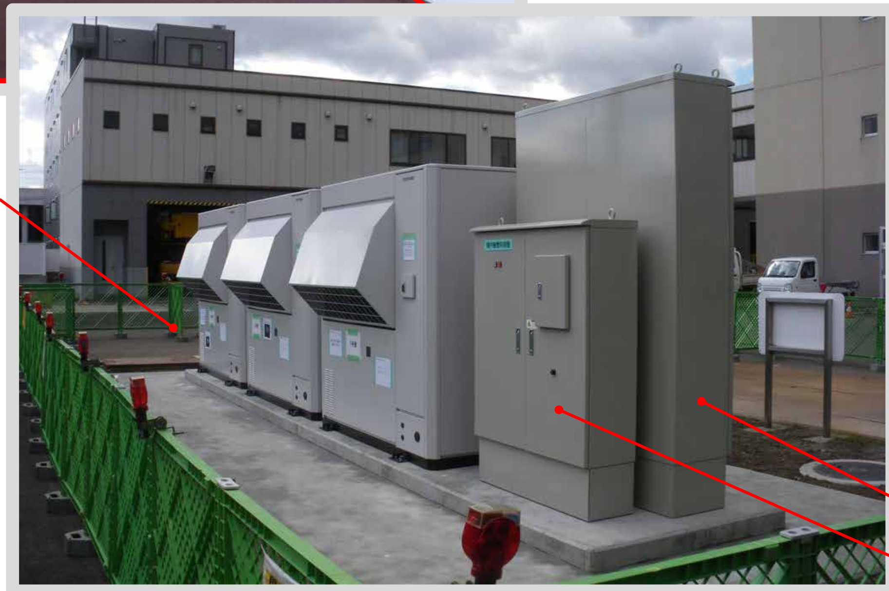
Heat pump unit
