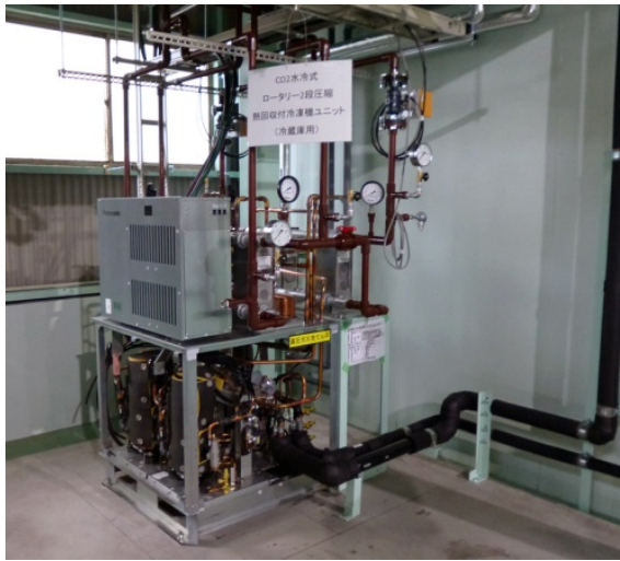
CO 2 20HP water cooling refrigeration system
