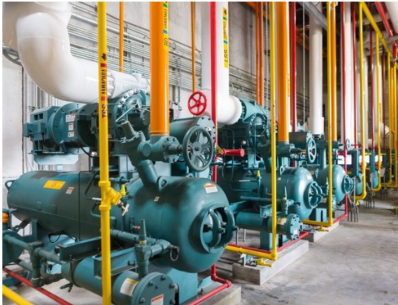
- AMMONIA MACHINERY ROOM -
