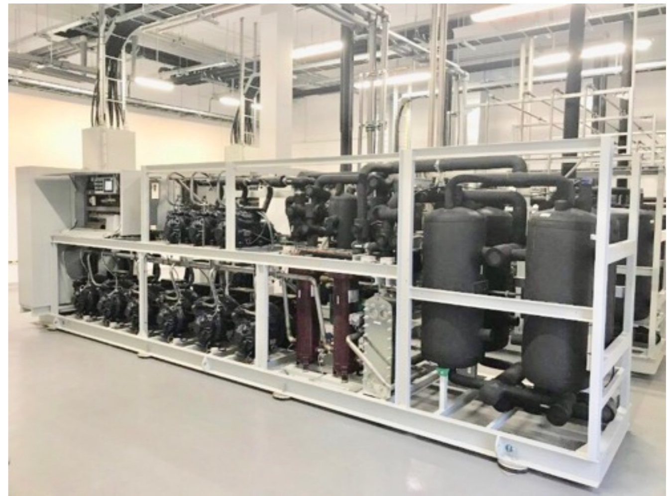
- CO 2 MACHINERY ROOM -
