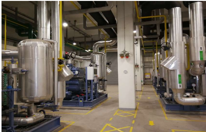
Packaged ammonia chiller in Taizhou factory
