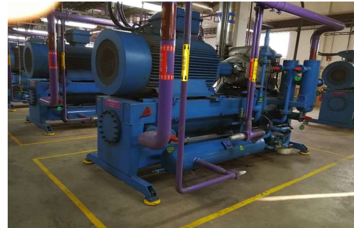
Ammonia refrigeration system in Tianjin factory
