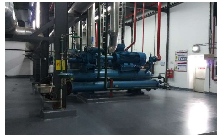
Ammonia refrigeration system in Shuangcheng factory
