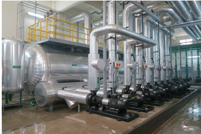
Centralized chilled water distribution system in Qingdao factory
