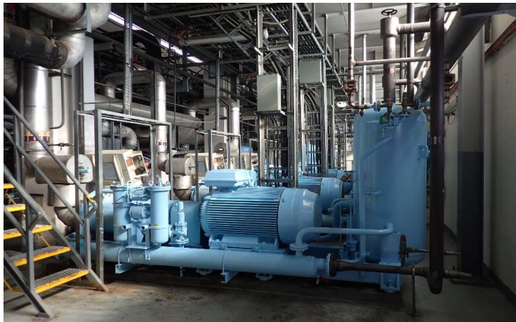
Ammonia refrigeration system in HongKong factory
