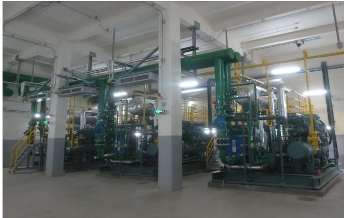
Packaged ammonia chiller in Qingdao coffee factory
