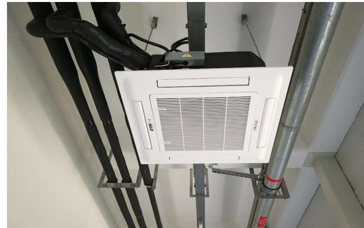
Chilled water fan /coil units used for offices
