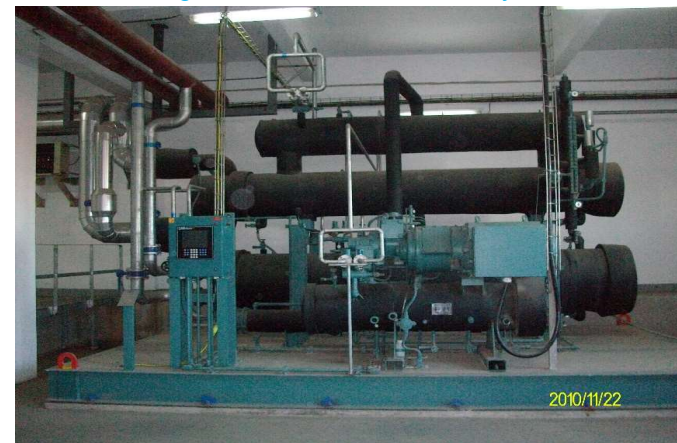
Packaged ammonia chiller in Tianjin water factory
