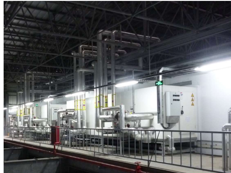
Co2 valve stations for cold store
