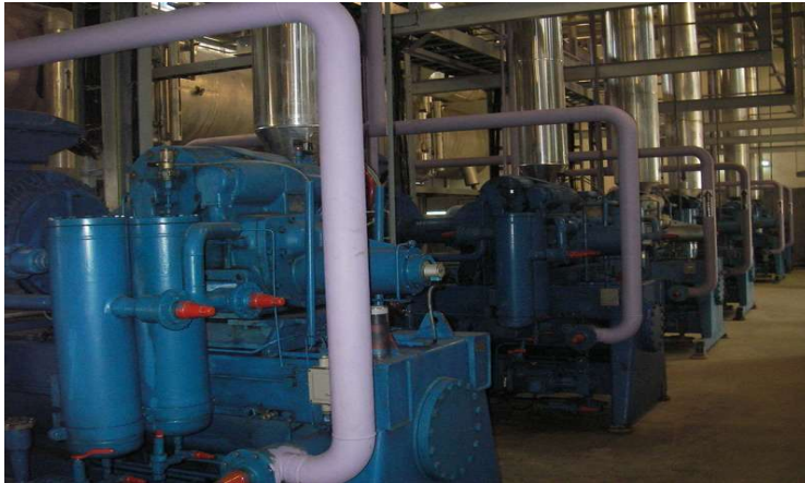
Ammonia refrigeration system in Guangzhou factory
