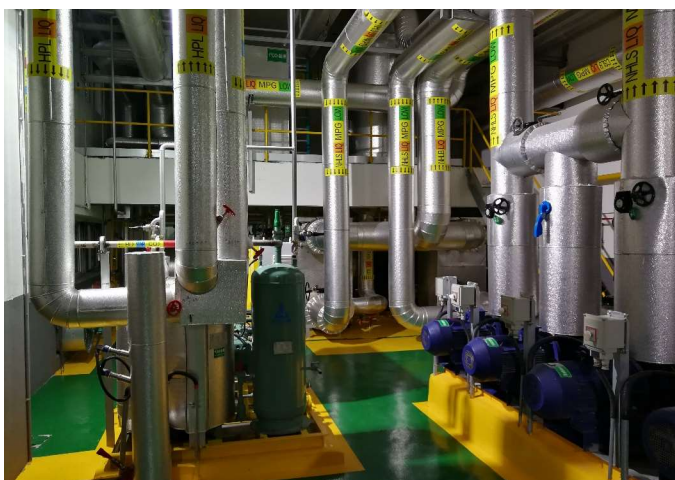
Overview of refrigeration plant room
