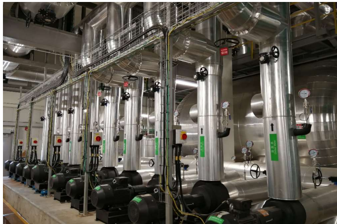
Centralized chilled water distribution system in Taizhou factory
