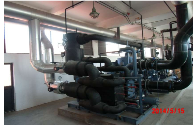
Packaged ammonia chiller in Shanghai TOTOLE FIRST factory
