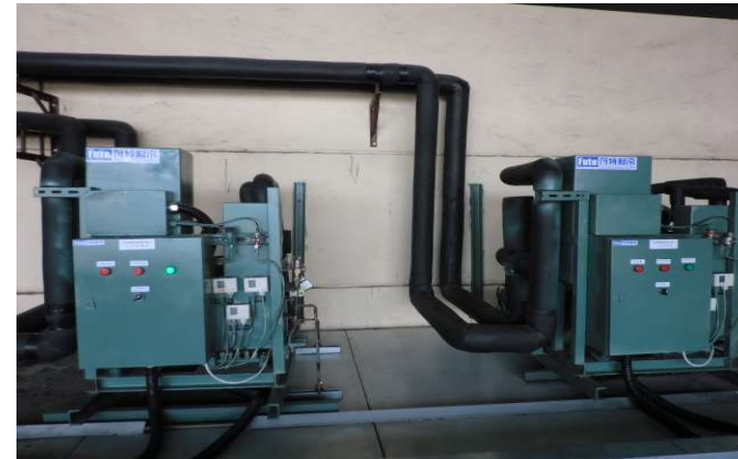
Co2 compressors /condenser cooled by 2°C chilled water
