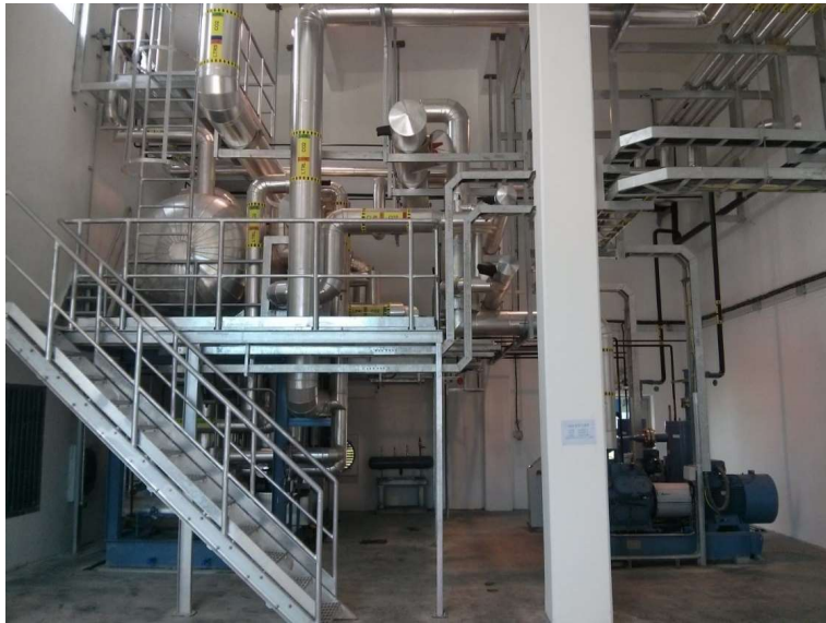
Co2 compressor room
