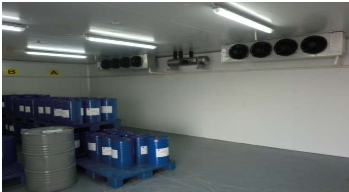
Co2 evaporators inside of cold rooms
