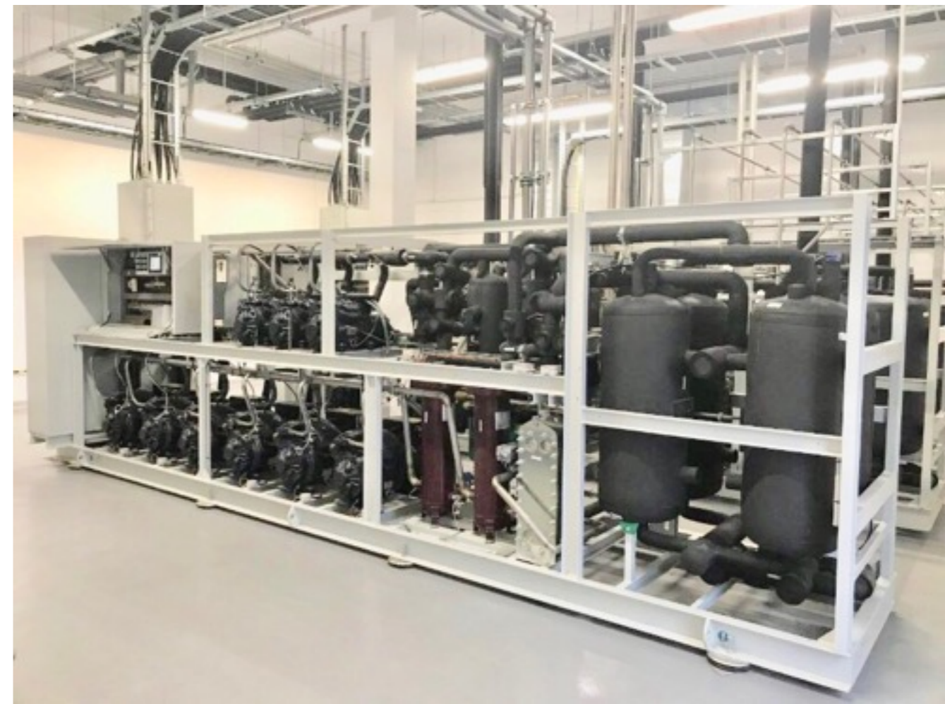
- CO 2 MACHINERY ROOM -
