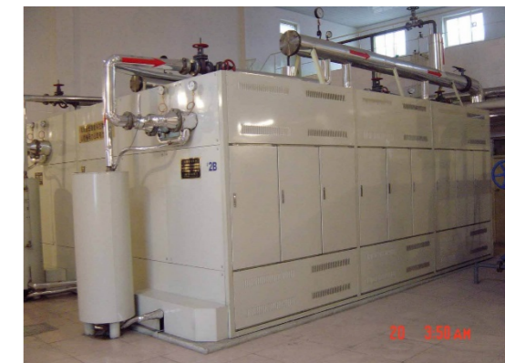
Coal-electricity: Heat Storage boiler
