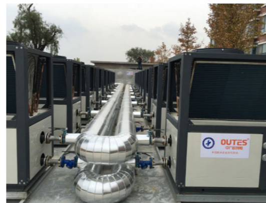
Coal-electricity: Heat pump centralized heating (town)
