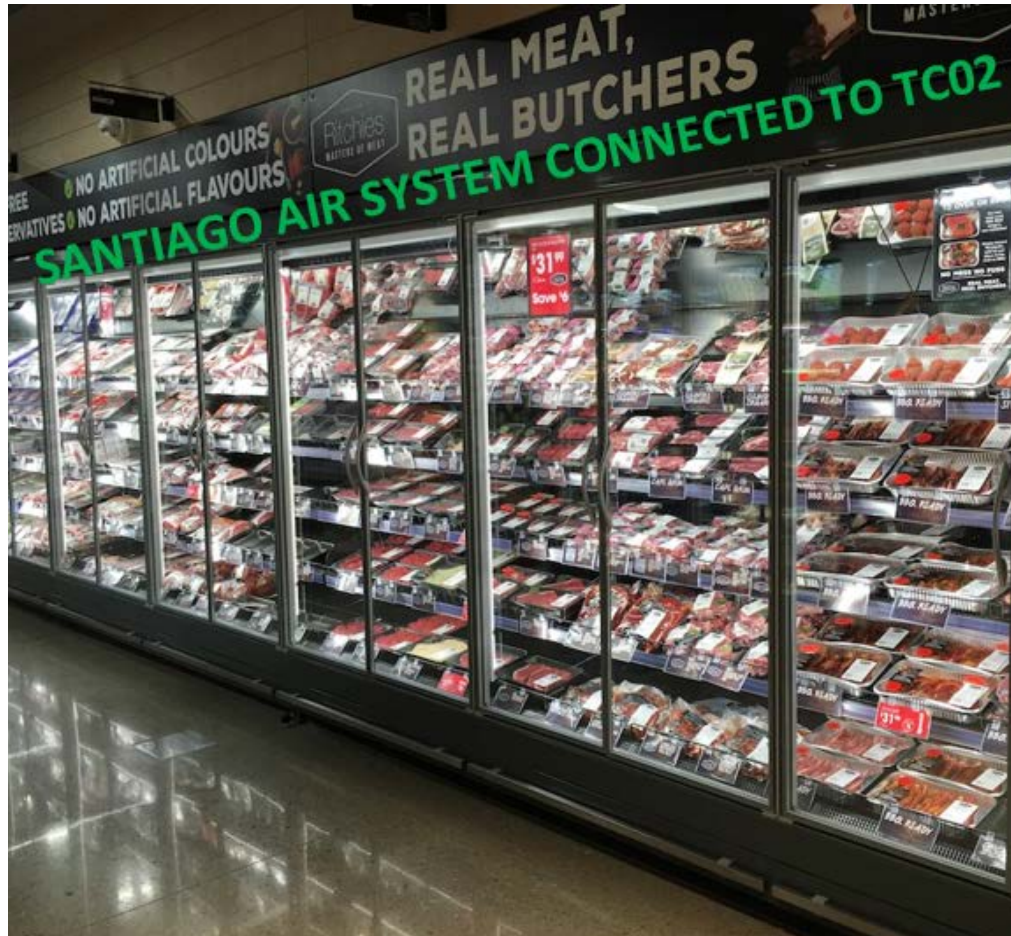
TC02 system at RITCHES IGA Beechworth, VIC
