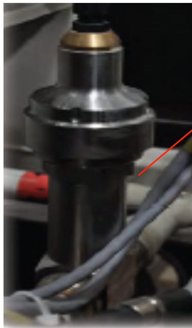
Flash Gas Bypass Valve
