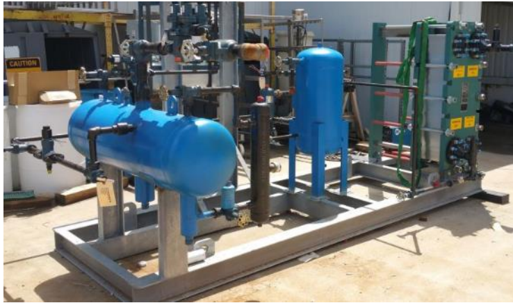
Low Charge RDC Package for Process Falling Film Evaporator – Nebraska, Phase I
