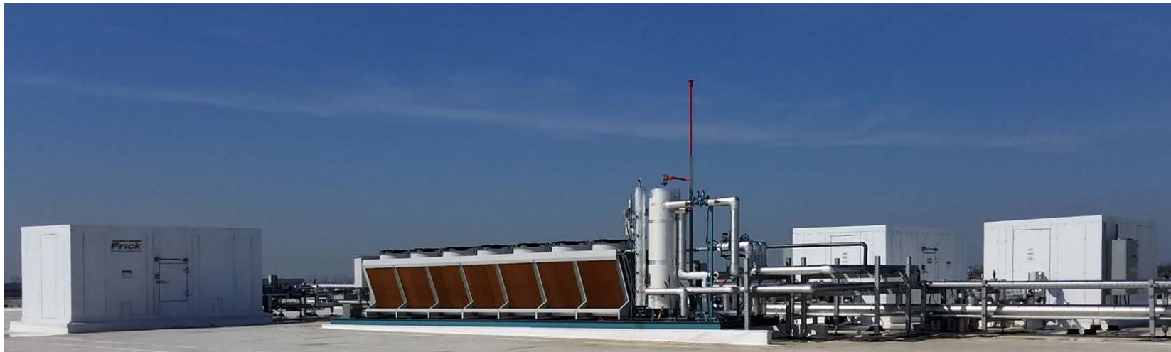
RDC #3 Servicing the Freezer/Cooler #4 and 1/2 Freezer #3
