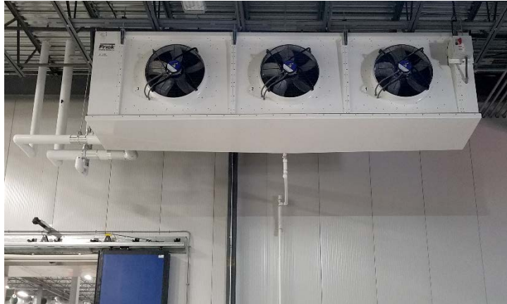
Loading Dock Evaporator
