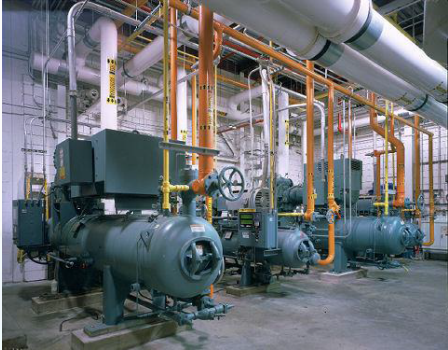
Large pumped system
