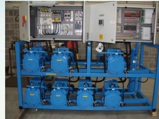
Large centralised pack
