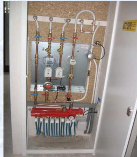
Heating and cooling water measurement station
