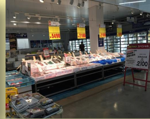
Open Chilled Room
